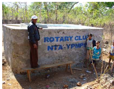
Concrete 15,000 litre off-roof water tank
